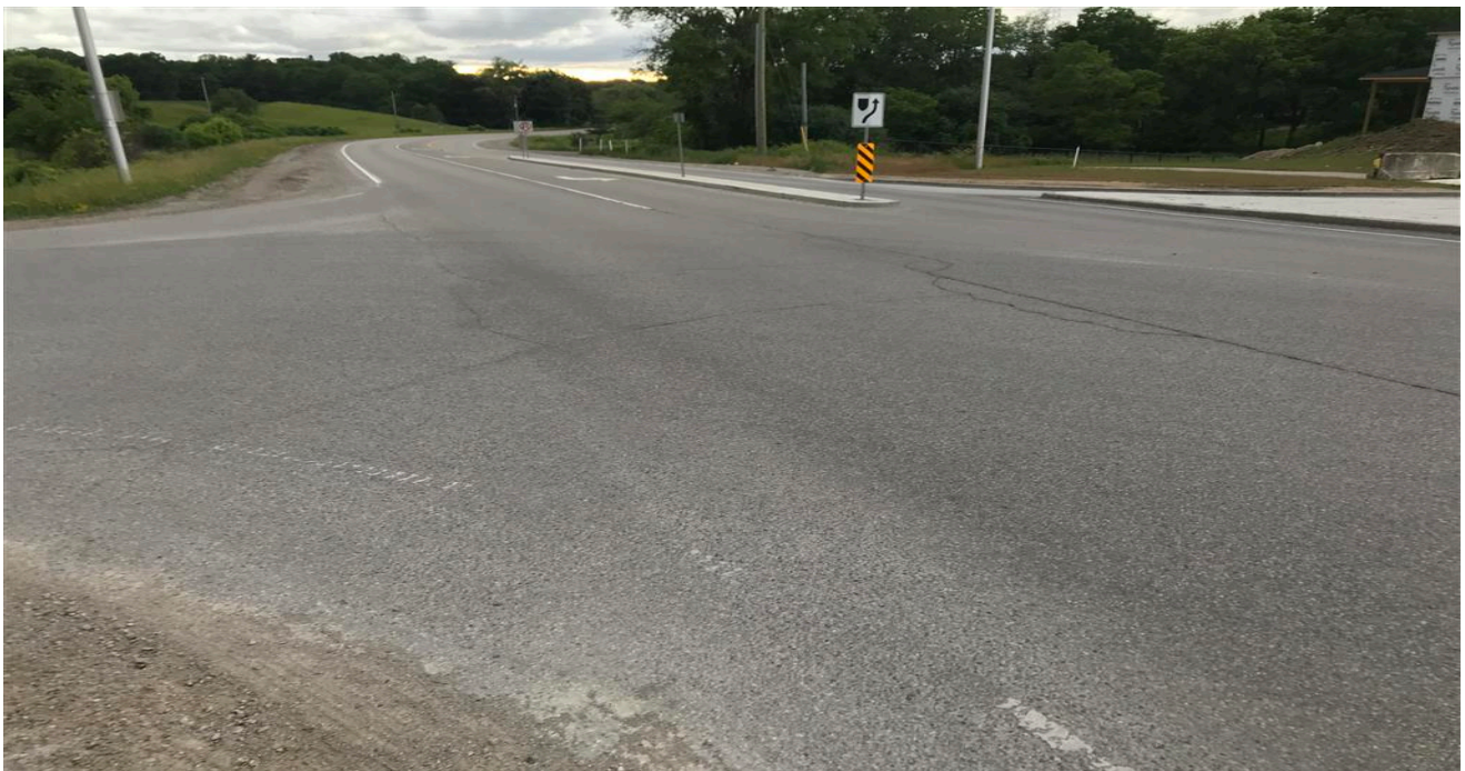
Photograph 2: Oxford Street West and Gideon Drive intersection, looking west. Note longitudinal cracks.
