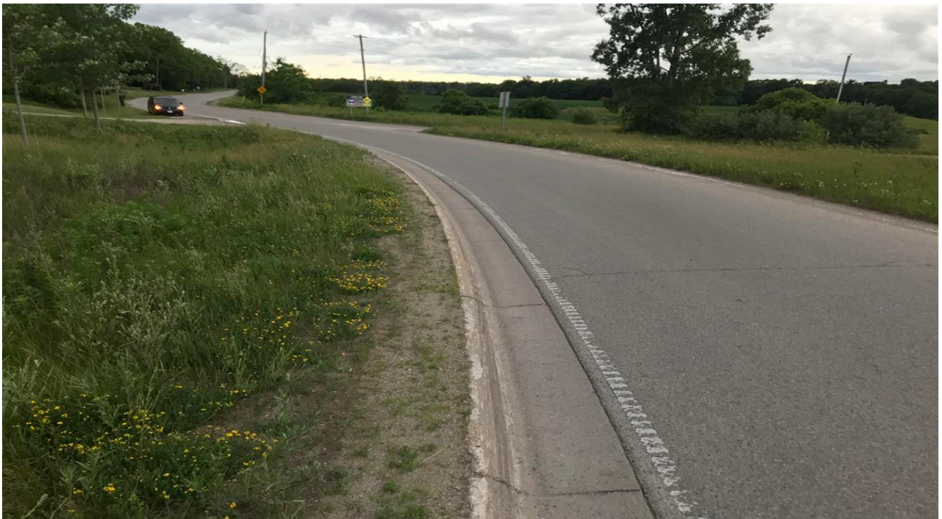
Photograph 4: Gideon Drive N/E ramp lane to Oxford Street West, looking southwest. Note transverse cracks.
