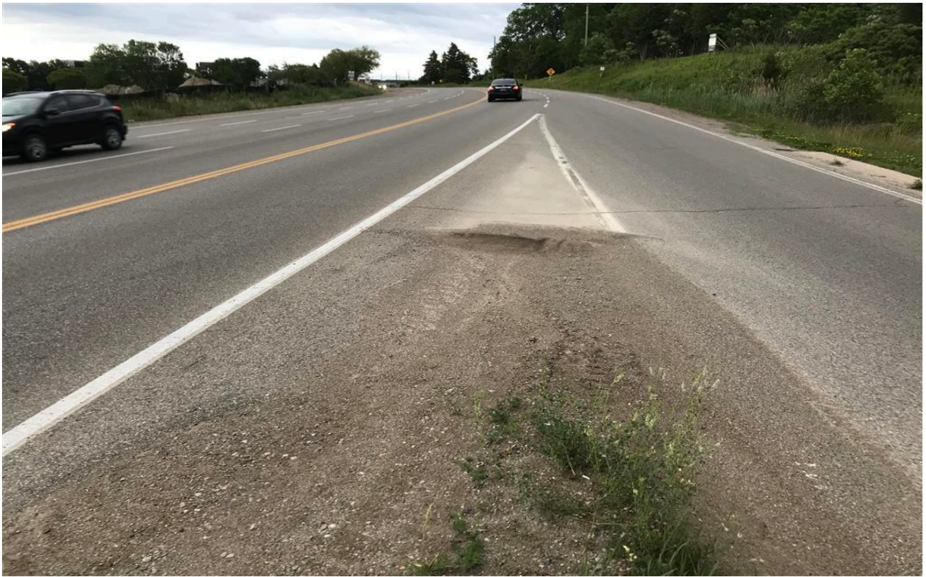
Photograph 3: Oxford Street West and Gideon Drive intersection, looking east. Note transverse cracks.
