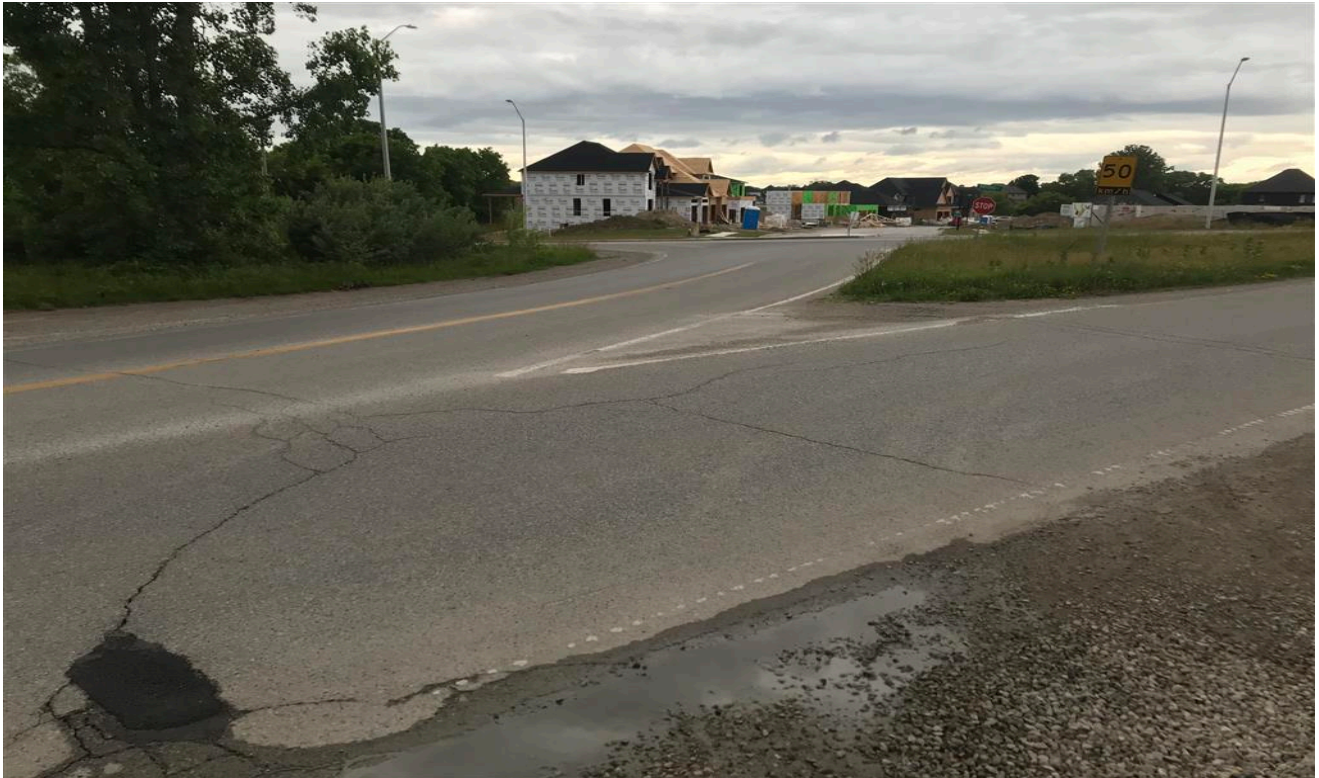
Photograph 1: Gideon Drive, south gravel shoulder, looking north to intersection. Note alligator and edge cracking of eastbound lane and transverse cracks.
