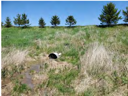
Photo 35: Location 13 – Outlet Pipe From Pond 1
