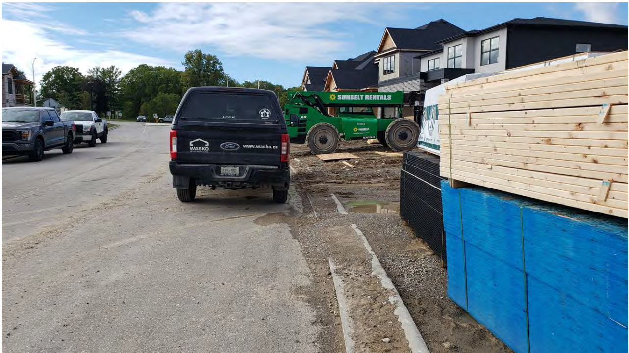
Image 14: A representative example of the disturbed Kains Road ROW; facing south, September 24, 2021.
