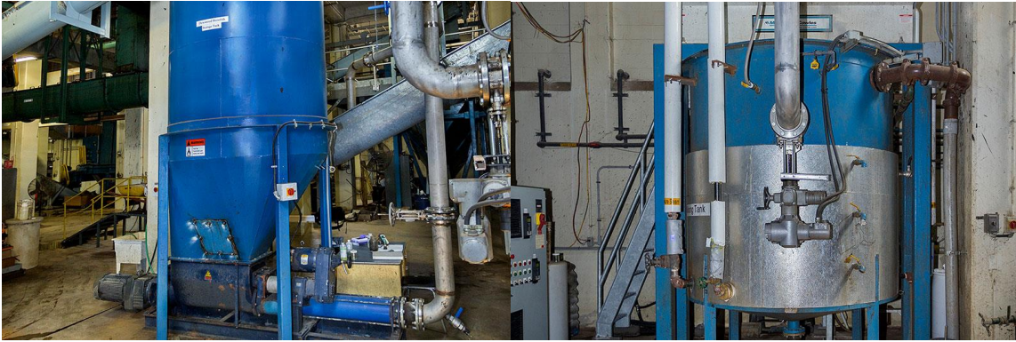
Figure 8. Photos of the Lystek facility operated at the Guelph Wastewater Treatment Plant (Courtesy: https://lystek.com/projects/guelph/ )
