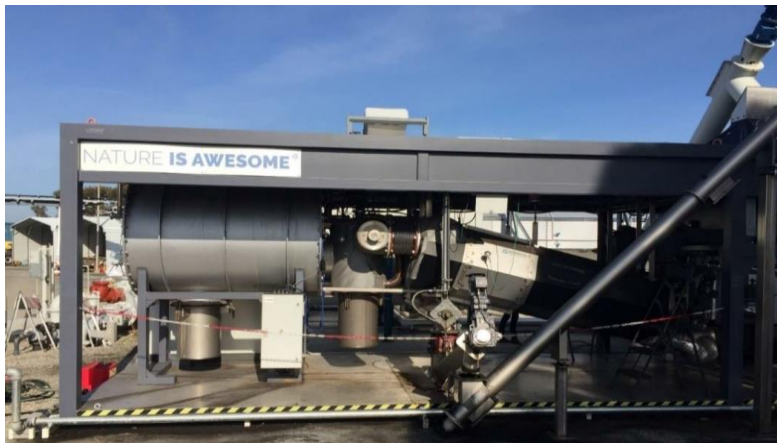
Figure 7. Example of a sludge-to-fuel process operated at the Silicon Valley Clean Water Agency Water Resource Recovery Facility in Redwood City, California
