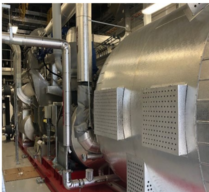
Figure 12 ORC Engine at Greenway WWTP
