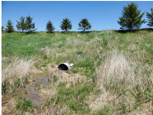
Photo 35: Location 13 – Outlet Pipe From Pond 1
