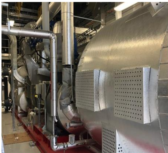
Figure 12 ORC Engine at Greenway WWTP
