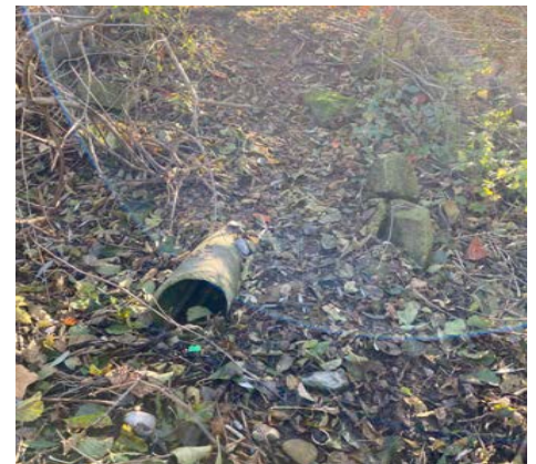
Figure 14: Existing Pipe Sticking out of Footpath
